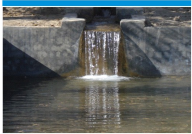
Water Reservoir getting filled from the water channel lined with reservoir from rehabilitated Karez by ADPB in flood affected Regora UC of Ziarat funded by AUSAID (snapshot by senior engineer of ADPB on 8 Dec 2011)
